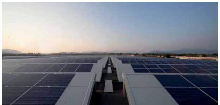
Photovoltaic roofing of the Company
