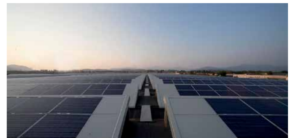
Photovoltaic roofing of the Company
